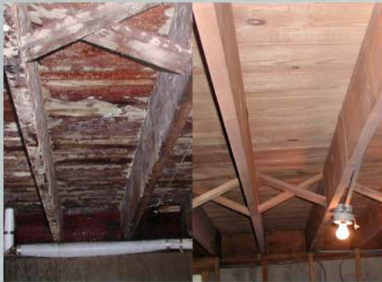
Mold removed from delicate wood surface
